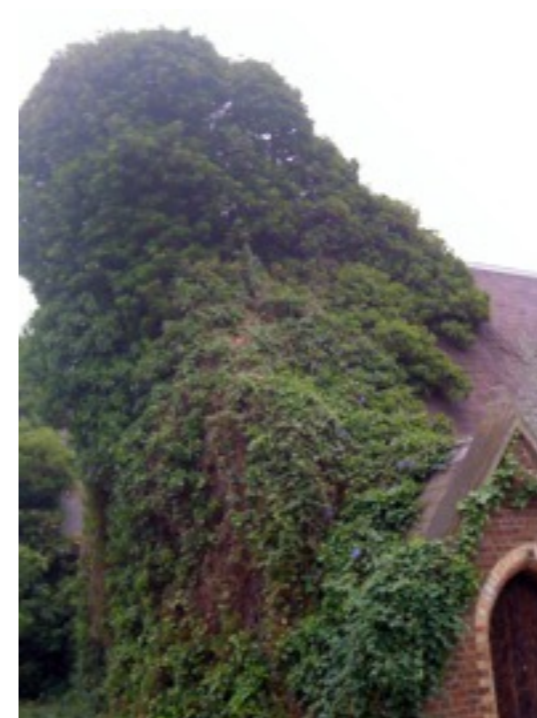
A tree and vines grow from the roof and walls of a church. Melbourne, Australia.
